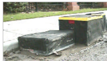
Street view – FilterBales stopping sediment run off at a new residential building development
